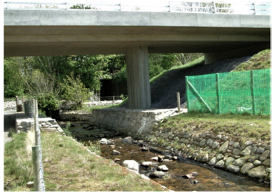
Figure 8. Open-span bridge taking a re-routed river under a new road. Temporary fencing is used to guide R. hipposideros under the structure until new hedgerow planting is established. Bethesda Bach Bridge, A487 Llanwnda, Wales, UK. © J. Matthews.
