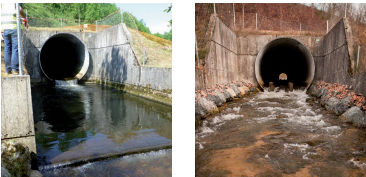
Figure 4: Downstream exit of the culvert before (left) and after (right) the adjustment works.
